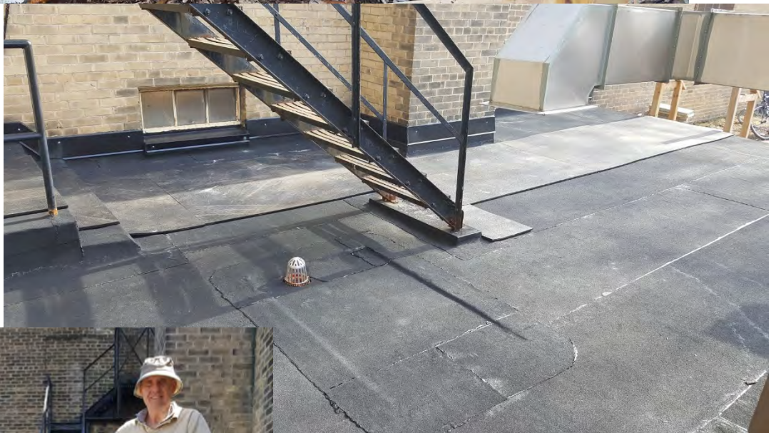
New boiler roof completed, rubber mats for walking, drain under fire escape.
